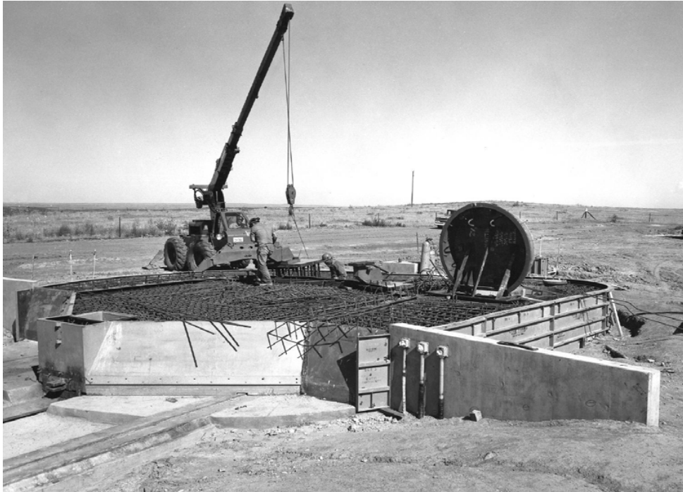
Plate 34. Launch Facility nearing completion in South Dakota (Courtesy of Peter Kiewit and Sons', Inc.)
