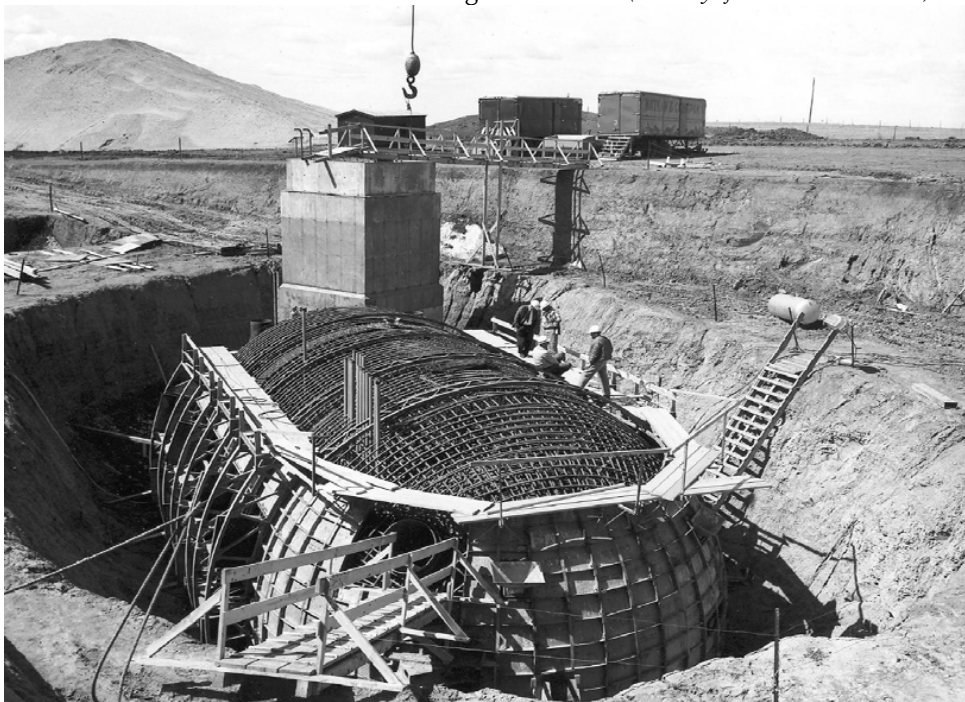
Plate 29. Launch Control Center under construction in South Dakota (Courtesy of Peter Kiewit and Sons', Inc.)
