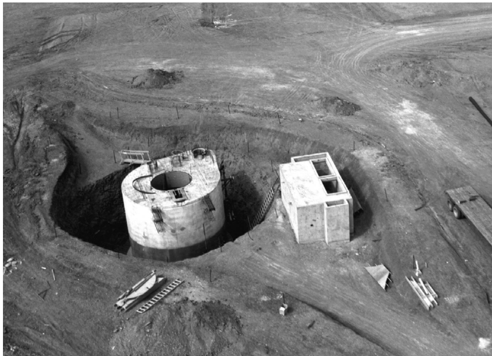
Plate 33. Aerial view of a launch tube under construction in South Dakota (Courtesy of Peter Kiewit and Sons', Inc.)
