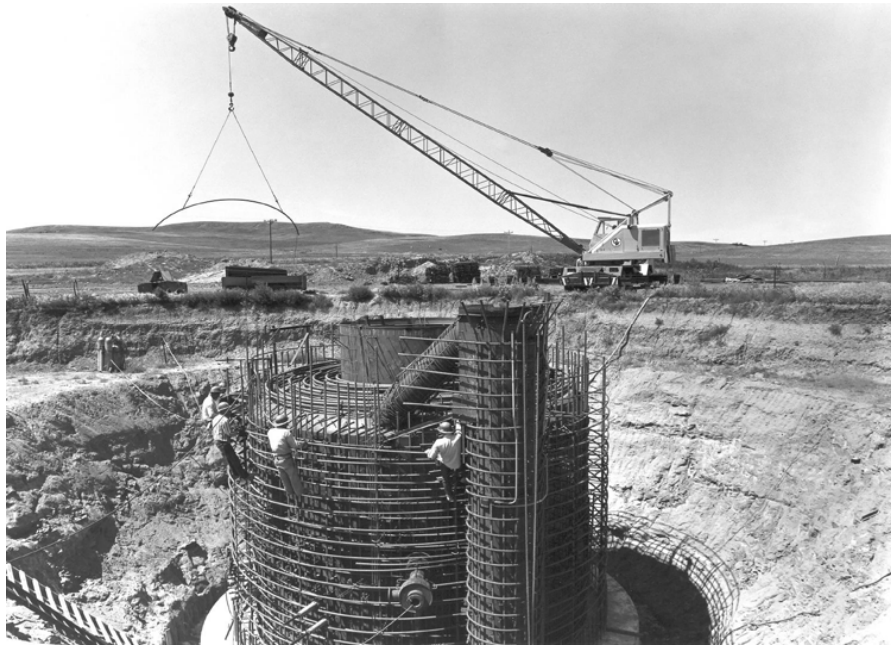
Plate 32. Launch tube under construction in South Dakota (Courtesy of Peter Kiewit and Sons', Inc.)
