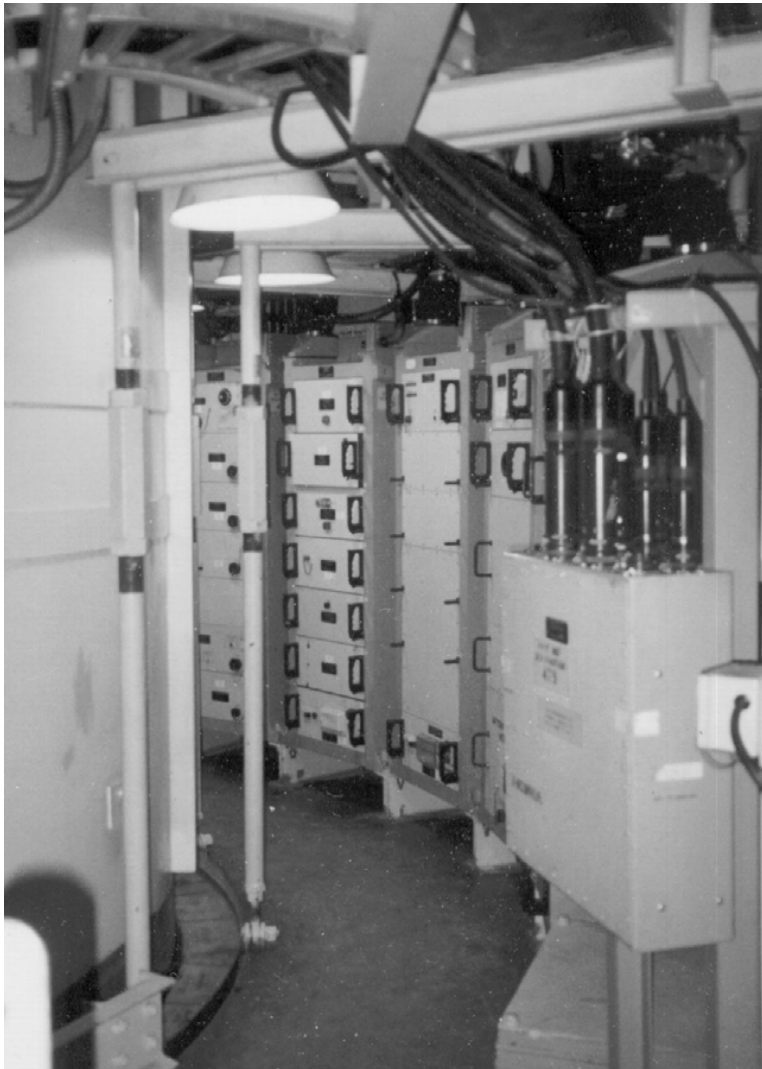
Plate 53. Interior of Delta- 09 silo showing launch tube encircled by electronic equipment (Courtesy of National Park Service, Photograph by Richard M. Kohen)
