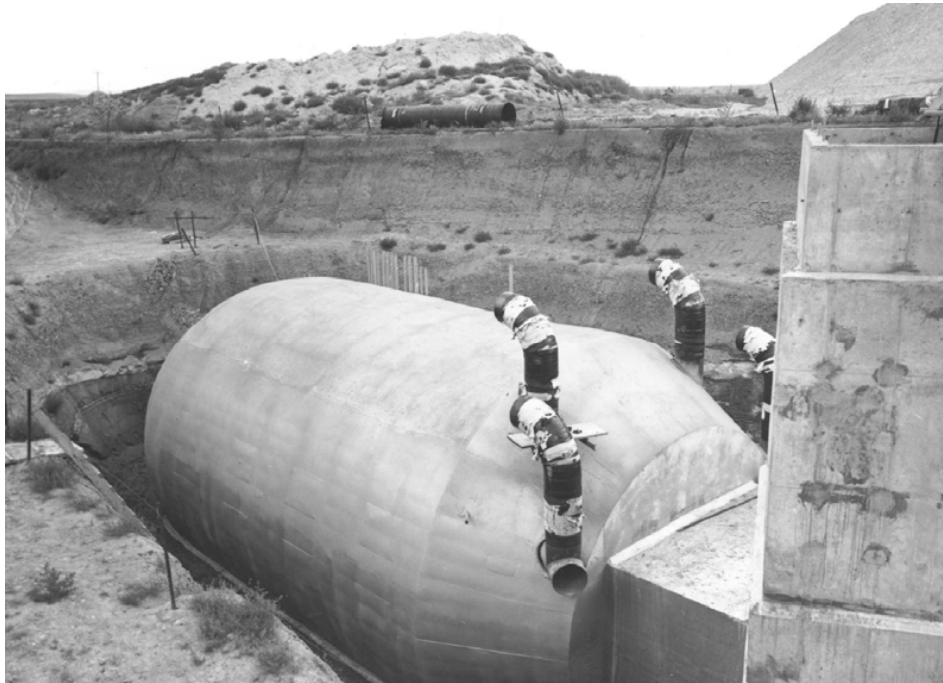
Plate 30. Launch Control Center nearing completion in South Dakota ( Library of Congress, Prints and Photographs Division, Historic American Engineering Record, Reproduction Number HAER SD- 50- 30 )
