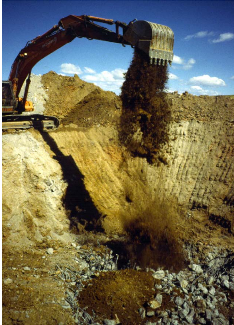
Plate 79. Missile silo being filled after implosion, South Dakota (Courtesy of the 28 th Civil Engineer Squadron, Ellsworth Air Force Base)
