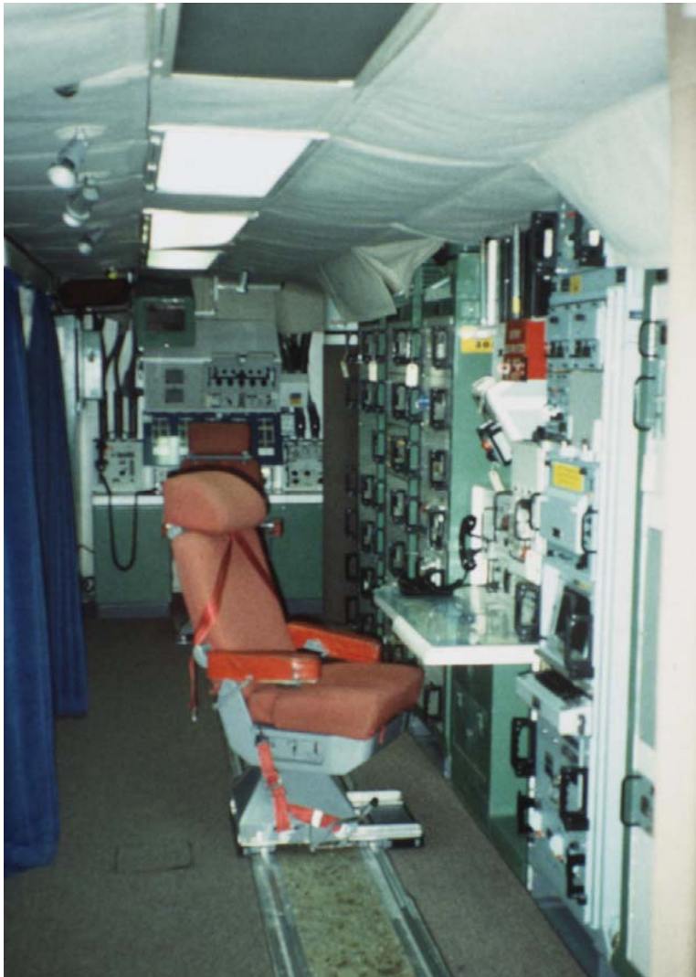
Plate 45. Launch Control Center at Delta- 01 (Courtesy of the 28 th Civil Engineering Squadron, Ellsworth Air Force Base)
