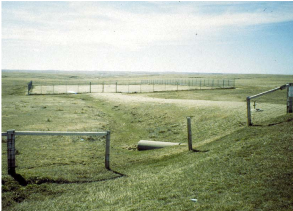
Plate 8o. Launch Facility after completion of deactivation, South Dakota ( Courtesy of the 28 th Civil Engineer Squadron, Ellsworth Air Force Base )
